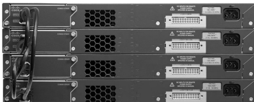
Figure 5. Cisco FlexStack-Plus switch stack
